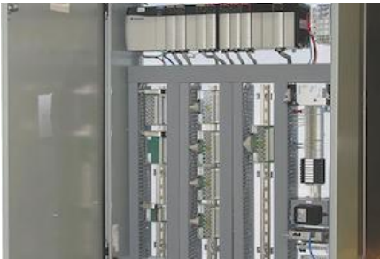
Control Panels & Systems
