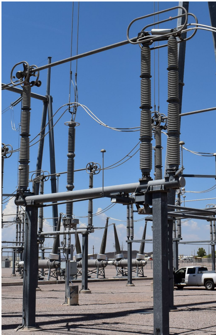
Figure 1 An example of a switch in a switchyard.
